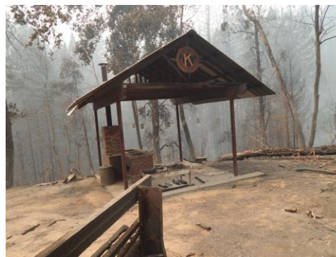
Severe but reparable damage to the dining shelter
